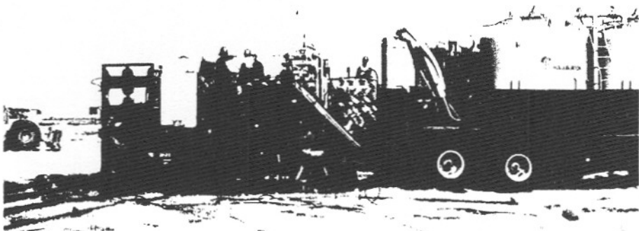
Fig. 3. Pumping equipment for operating this abrasive jet cutting system is massive, but common to oil fields all over the world.
